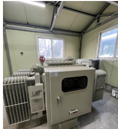
Photo of temporary power transformer installed
