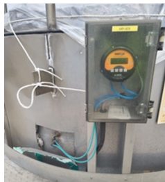
Photo of digital differential pressure gauge installed
